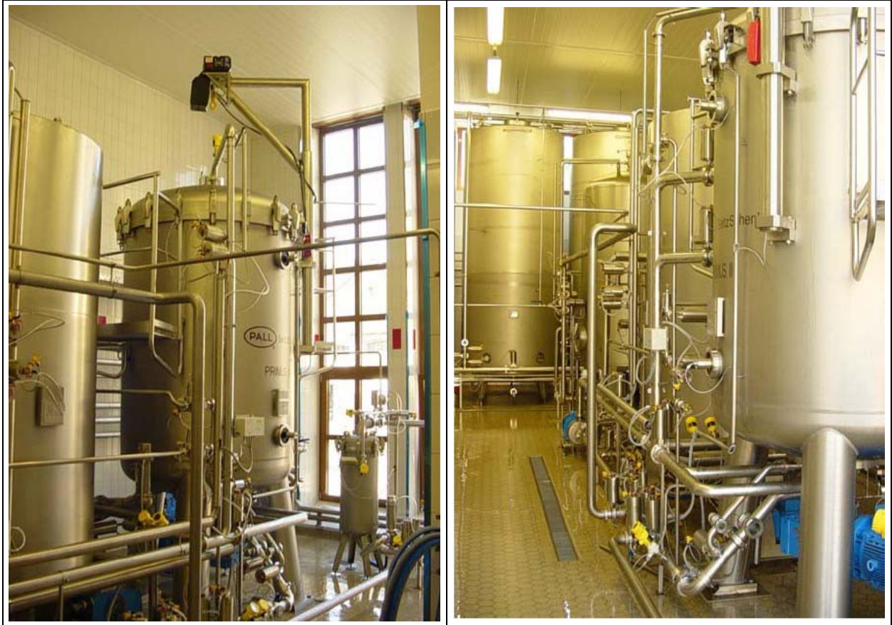
Filterline with the ZHF Primus III D.E. filter for re-generable filter aids, and the storage tank as well as CIP Tank in the Altenburg Brewery
